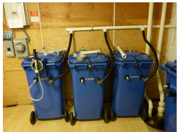
Fig. 3. Full bins connected to aeration
